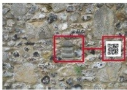
Voussoir, originally forming part of an arch, reused in an inverted position in the west wall, with associated QR code
